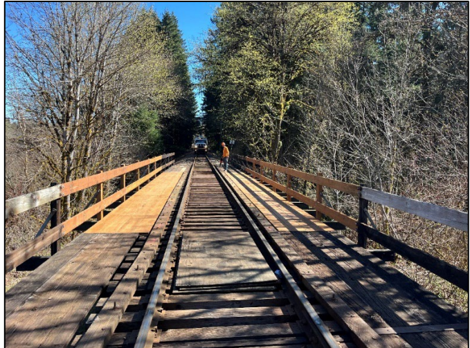
(Completed repairs to top deck of bridge, old decking and handrails had to be removed and were not salvageable)
