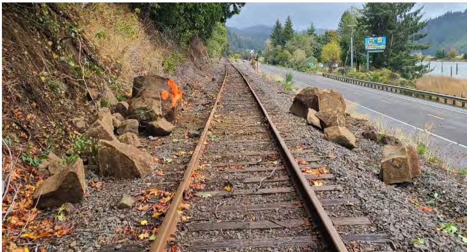
Photos: Before and after of downed boulders along Highway 126, cleared by the MOW team.
