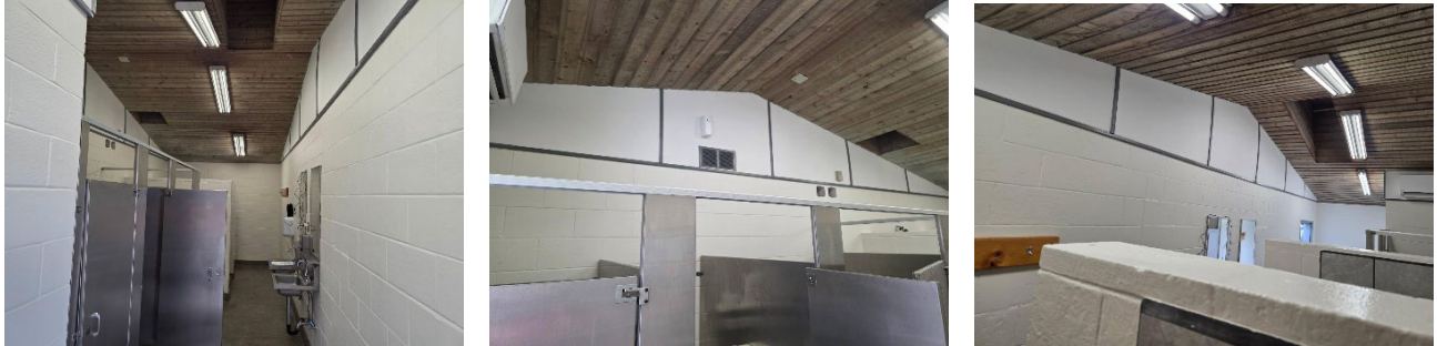
The finished look of the men’s restroom and showers at the RV Park.
