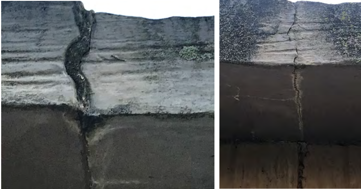
Gaps in the modular units that are needing resealed.
