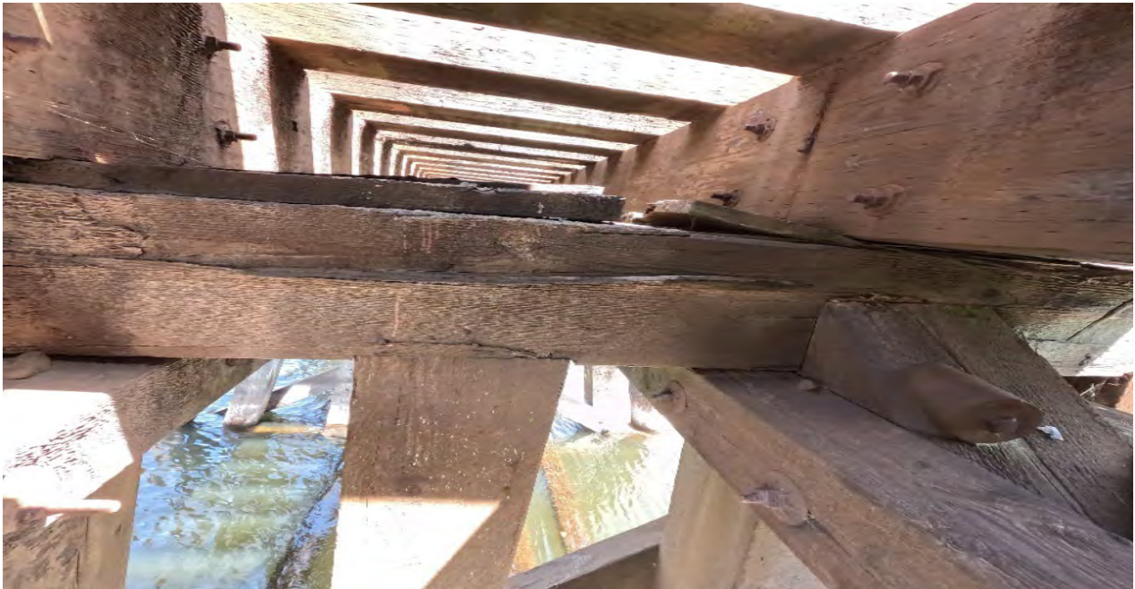
(Example of a failing cap before repair)
