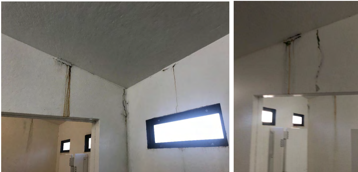
Leaks inside from the gaps in the modular units.
