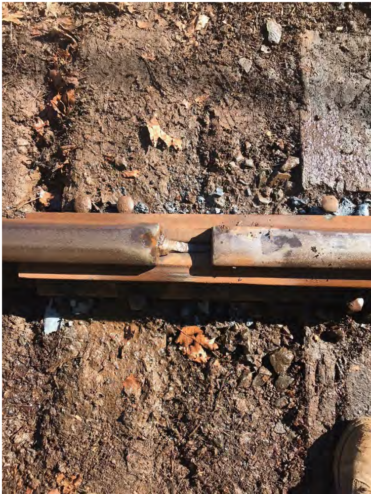
Example of broken rail in a joint.
