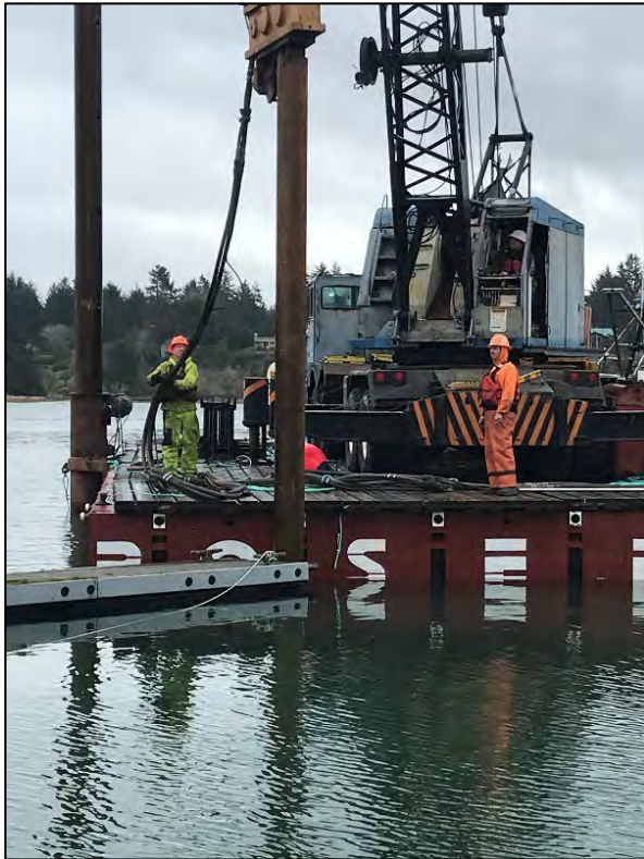
Billeter Marine use a vibrating head to drive a new 12” steel pile on D Dock
